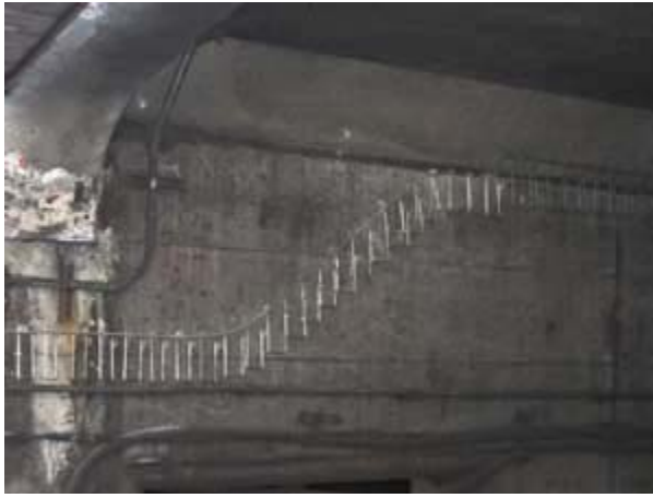
The new installation of the Rail Tray system above the existing messenger cable to be replaced.
